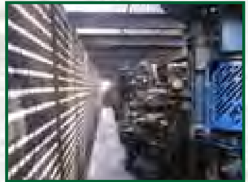
An example of an underground well cellar with well heads. Matrix Oil Corporation
